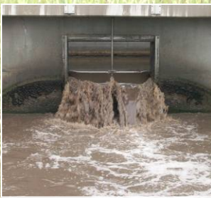
ReWa Water Treatment Plant
