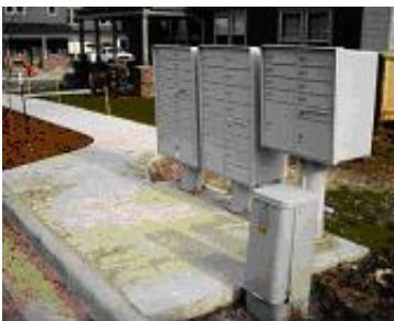
CORRECT – NOTE HOW MUCH CONCRETE WAS REQUIRED IN ORDER TO MEET LOCAL CODES
