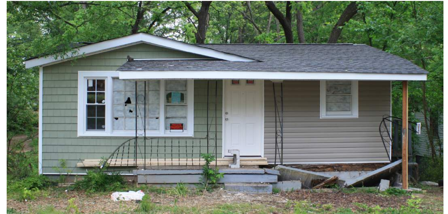
City View house with need of rehabilitation
