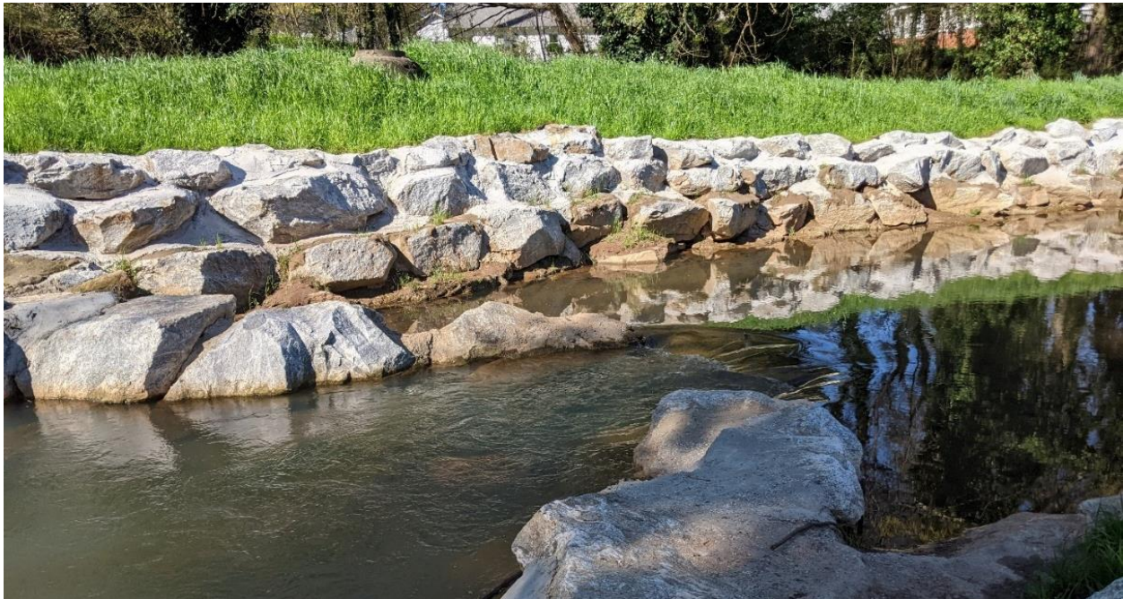
Figure 3.4 – Section of Brushy Creek restoration with cross vane and boulder wall armoring along a sewer line.
